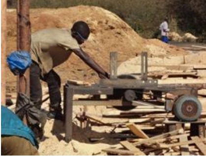
Picture 4: Workers in box production – with no saw guard
